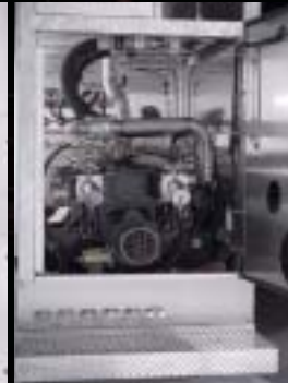
Full access to pump house
